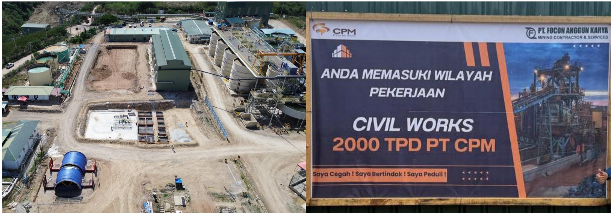
Figure 11. Carbon-in-Leach (CIL) gold processing plant expansion from 500 tpd to 2,000 tpd
