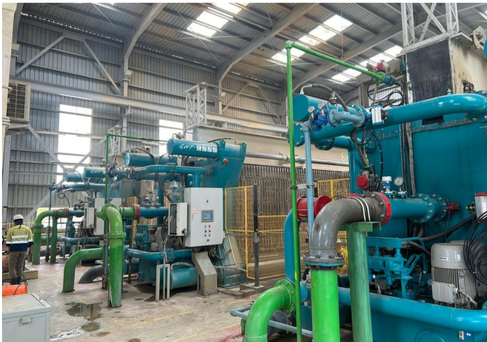
Figure 17. Filter-Press for Dry Tailing
